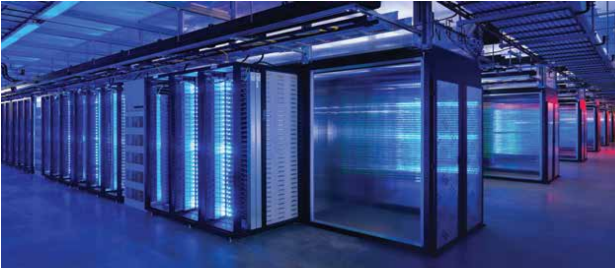
Figure 1 | Open Compute Project hardware in use at Facebook's Prineville, Oregon data center
